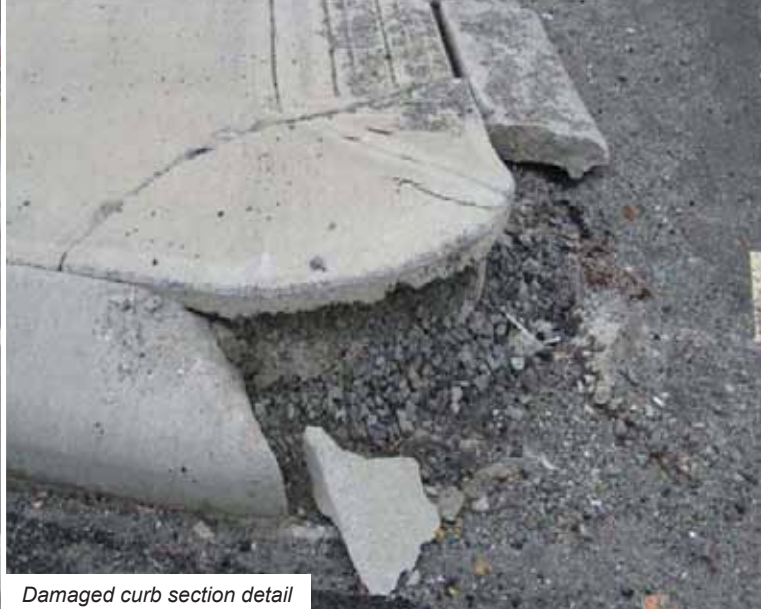
Damaged curb section detail
